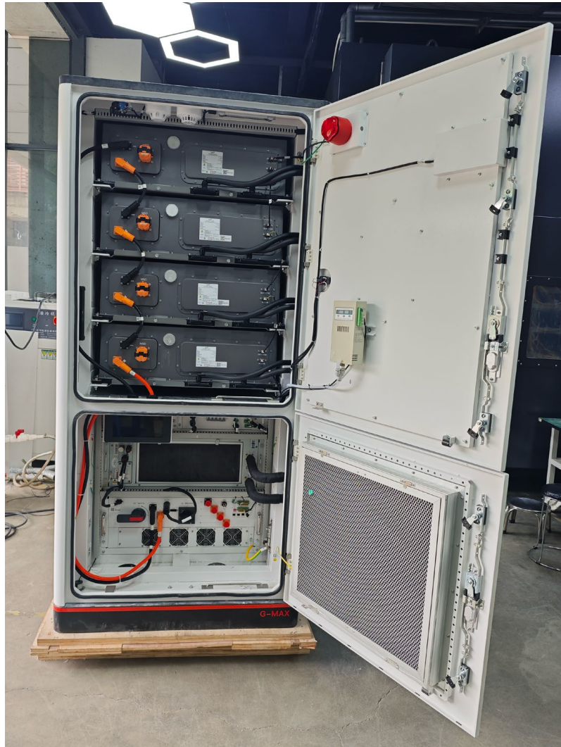
Inside view of battery system (with MSD)
