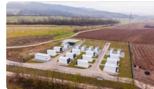
Trier, Germany 21MW/ 55MWh
