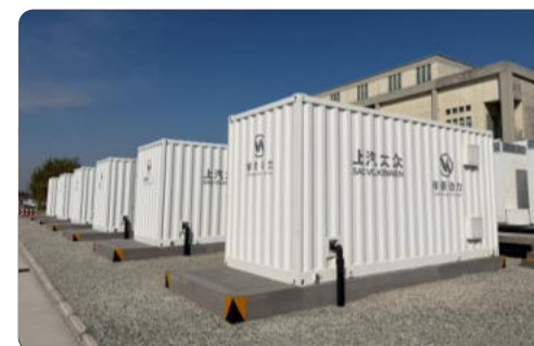
Ningbo, China 45MW/90MWh
