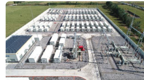
Shandong, China 100MW / 200MWh
