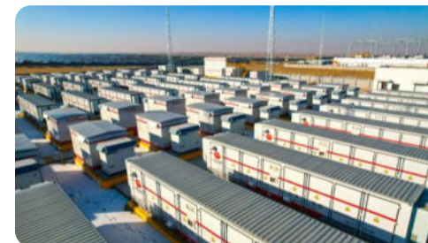
Ningxia, China 100MW / 200MWh
