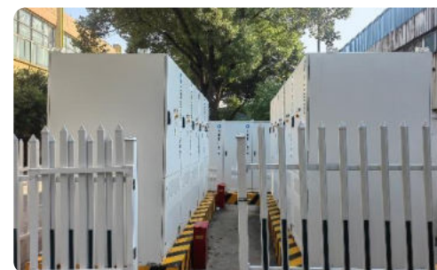
Zhejiang, China 1.25MW/2.61MWh
